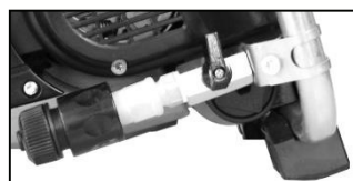
water supply closed (valve lever across)
